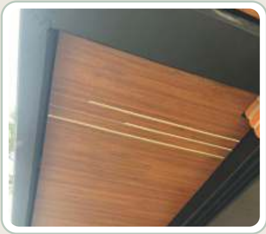
Fita LED embutida no forro
